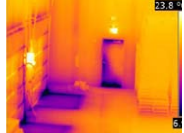
Cold air infiltration
